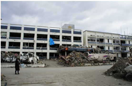
Figure 11. Damaged local government building
