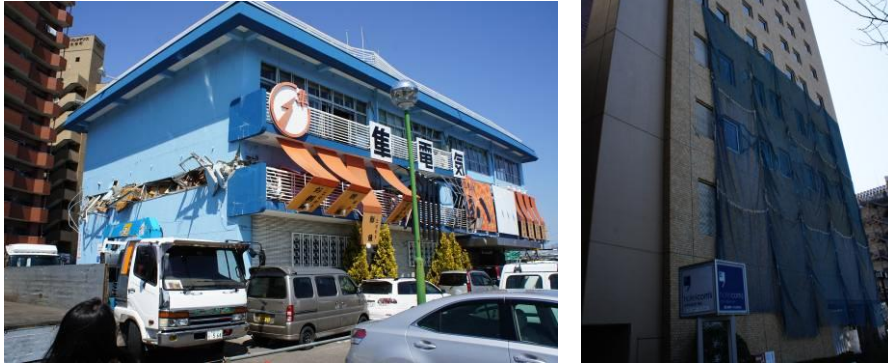
Figure 27. Building damaged by the earthquake
